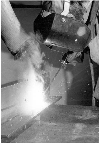
3.1 Manual metal arc welding with a covered electrode (photograph by courtesy of TWI).
